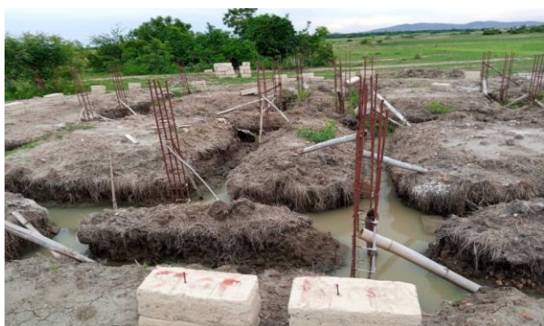
Fig. 2: A recent encroachment in the catchment that the Wildlife Division has halted. This is located at the northern part of the Muni lagoon close to the Ntakofa River. Source: Authors construct (2021)
