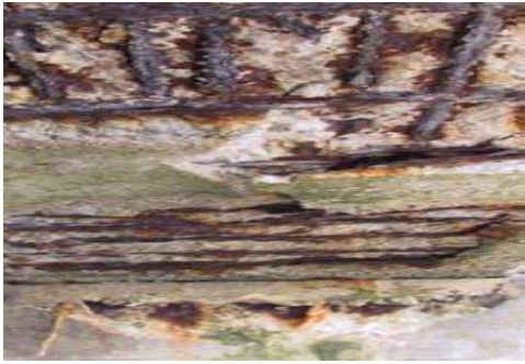
Fig. 6: Concrete cover was seen disintegrated from beams
