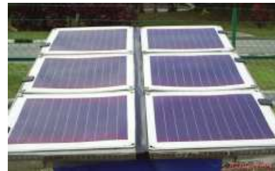
Plate 1: The a-Si modules used in System I.
